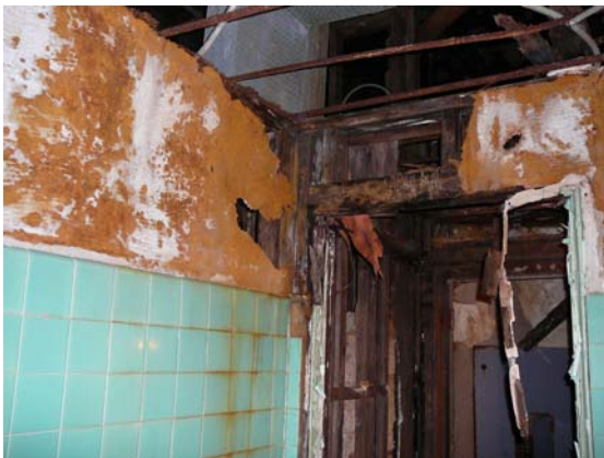
Failed plaster and rotting wood framing at entrance
