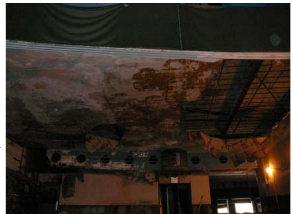
Failed plaster ceiling below mezzanine, note porthole diffusers
