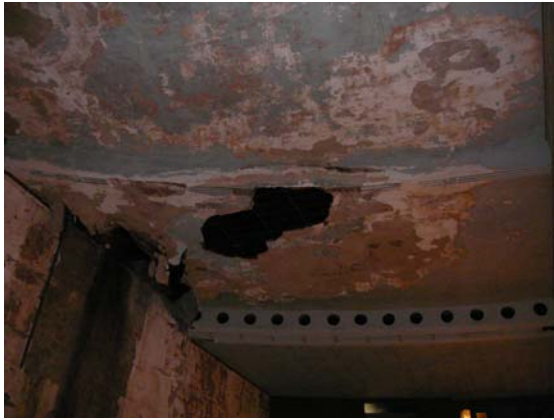
Failed plaster ceiling at east side of auditorium
