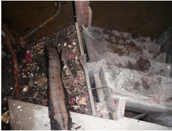
View of rotted platform and steps from stage
