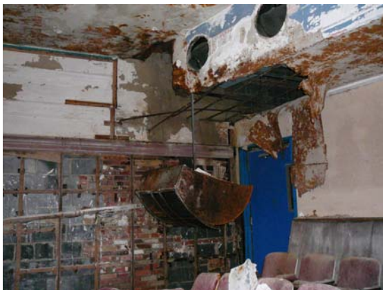
Mechanical soffit at rear of auditorium with hanging light fix-
