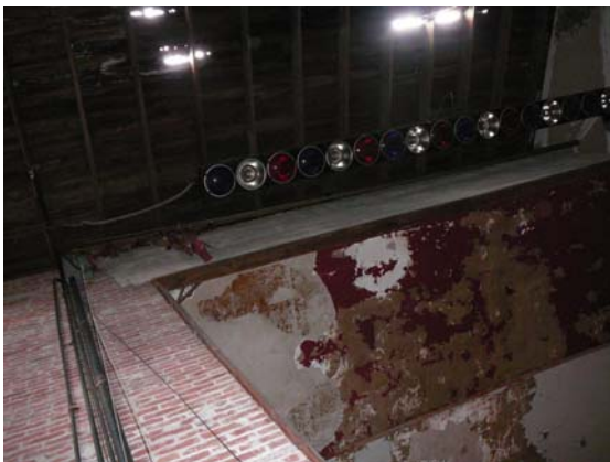
Remaining light fixtures over proscenium
