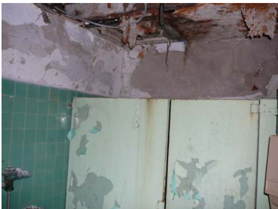
Rusted toilet partitions, failed plaster ceiling
