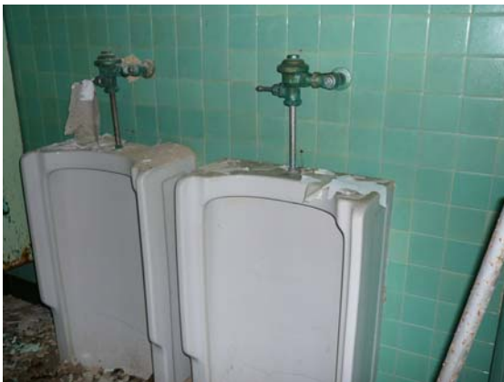
Floor mounted urinals
