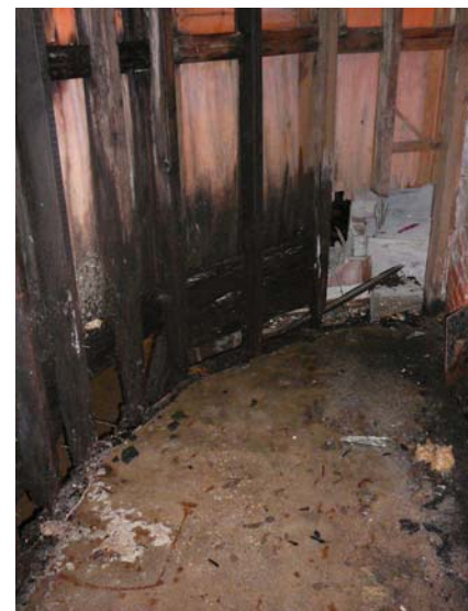
Rotted structure and veneer at small green room at stage east
