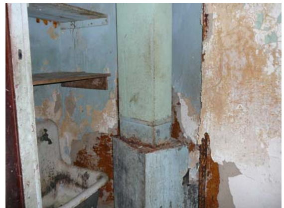
Mop sink and mechanical duct at Janitor's closet
