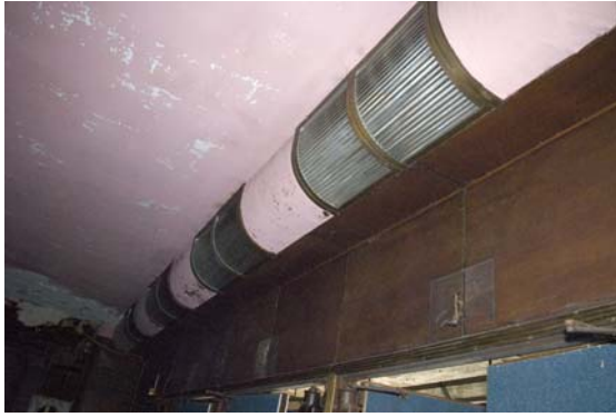
Glass rod light fixtures at soffit above lobby doors
