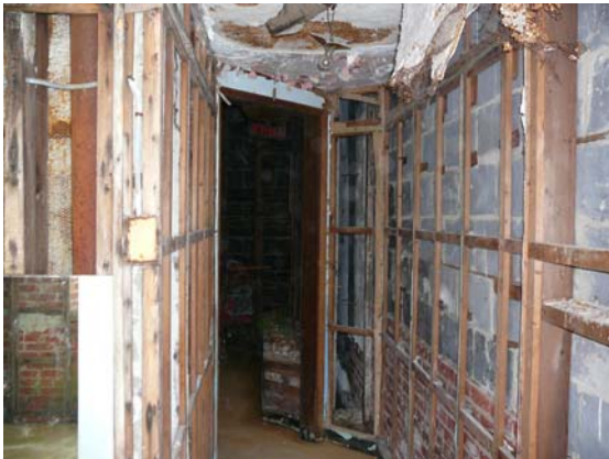
Access hallway to lounge, note missing paneled veneer
