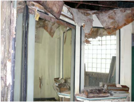
Triple mirrored wall at lounge, note failed plaster ceiling
