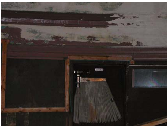
Original fire hose cabinet at front of auditorium
