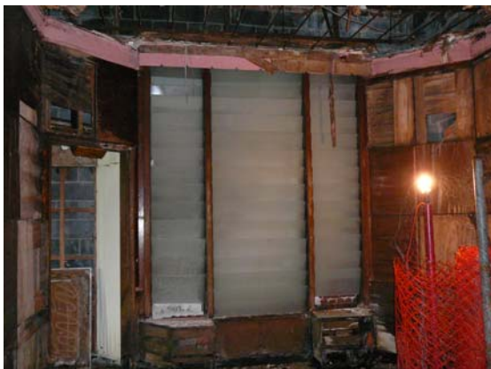
Backlit glass louver with planter box, note missing ceiling
