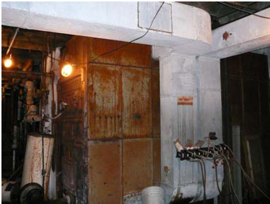
3. Main mechanical system
