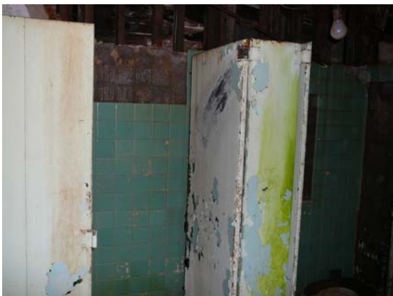
Rusted toilet partition and failed plaster wall at restroom
