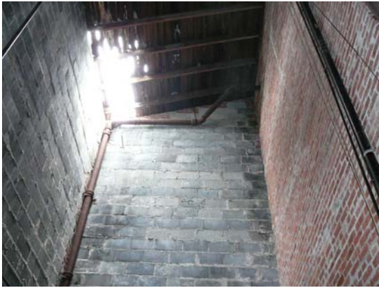
Failed roof system at fly gallery
