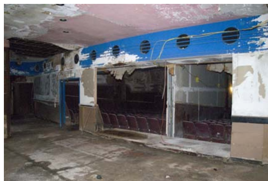
Inner foyer, note porthole soffit, missing ceilings and fifth build wall
