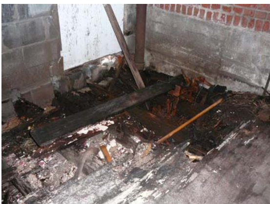
Extensive water damage at stage floor and structure
