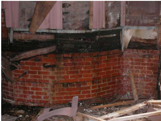
Vertical assembly with missing veneer, original trim remains
