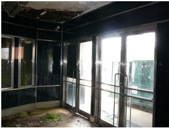
Exterior doors, note fire damaged ceiling and walls
