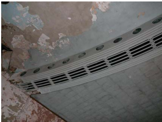
Mechanical diffusers and portholes at 2nd soffit step
