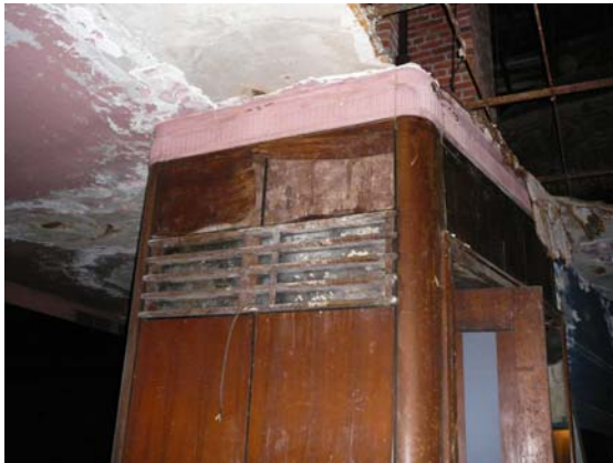
Wood veneered mechanical shaft, note failed plaster ceilings
