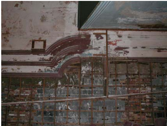
Plaster banding at sidewalls, note missing wood veneer
