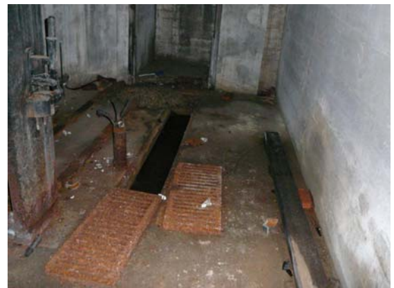
5. Electrical room below eastern restrooms
